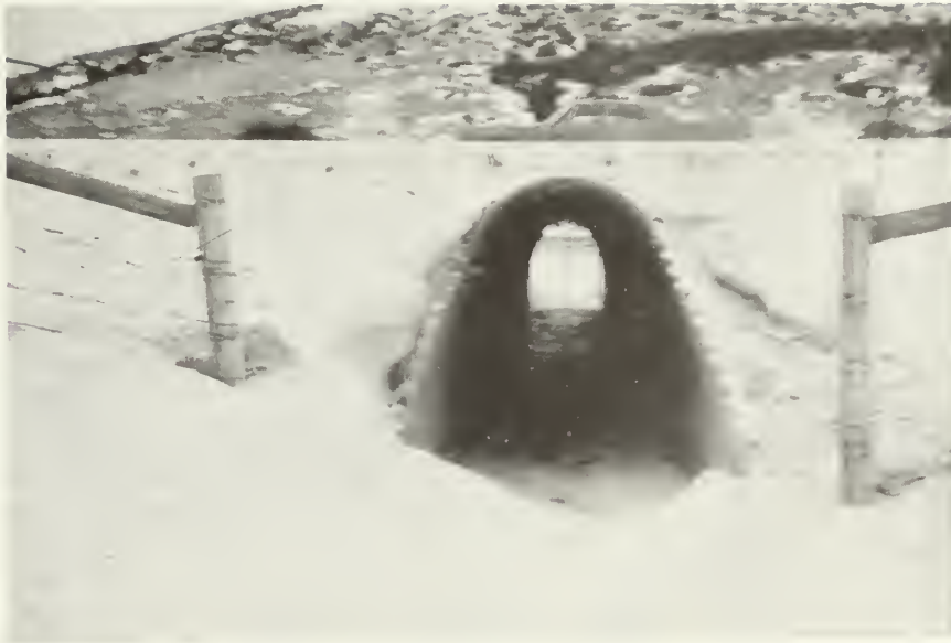
EAST ENTRANCE; photo taken 1/19/71 showing snow conditions, ice in pipe bottom.
